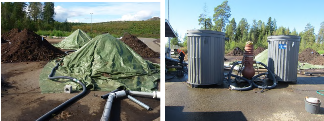
Figure 19. Odour abatement of the composting test heap by biofiltration system.
