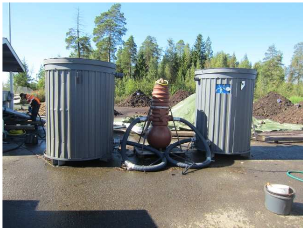
Figure 14-15. Odour abatement of the composting test heap by biofiltration system.
